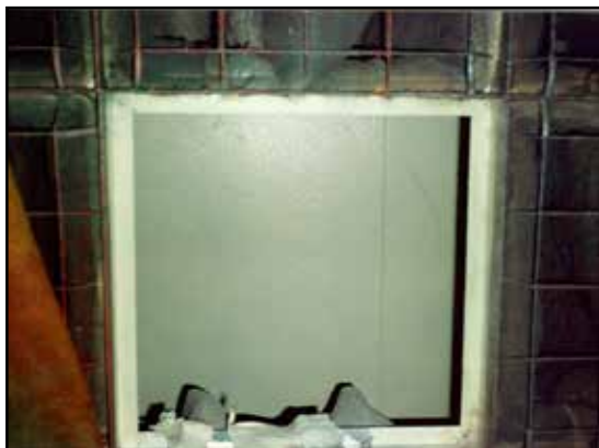
Clean Back Plenum
